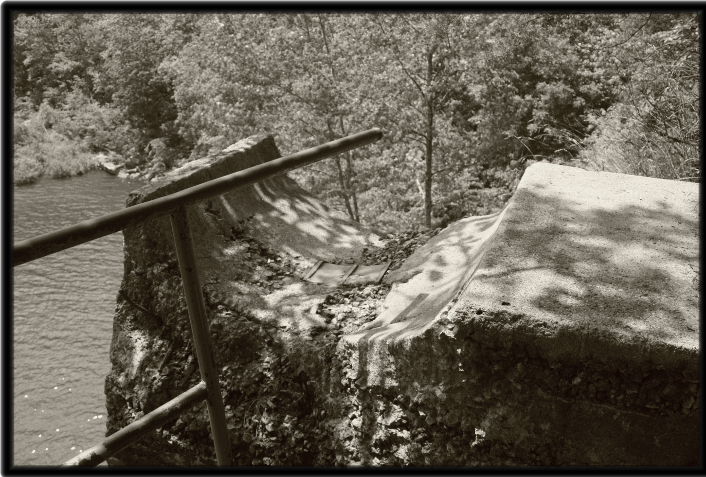
The 'cradle' for the pipe going down to the generator house at the base of the falls.
